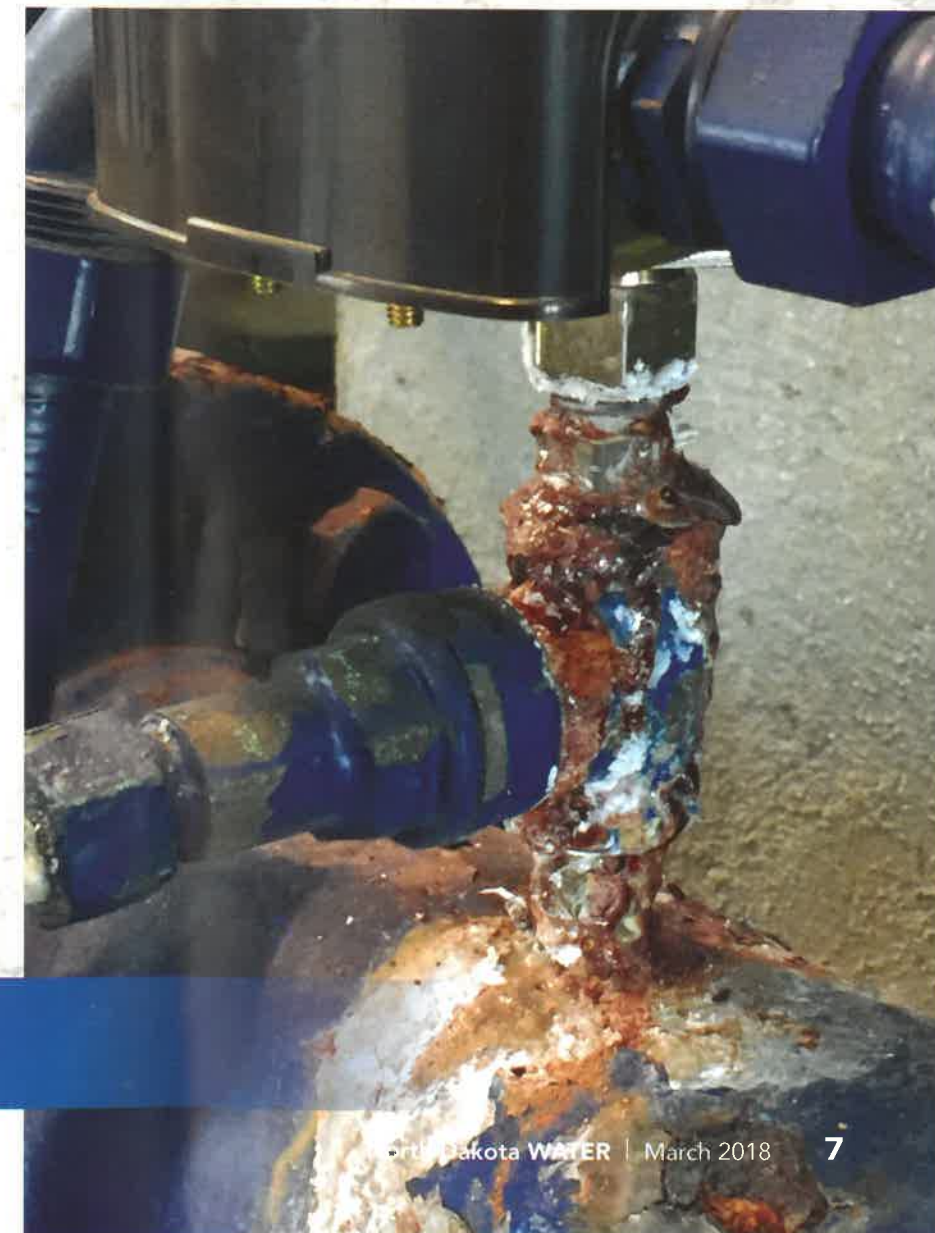
Poor water quality has caused corrosion issues in the distribution system.
